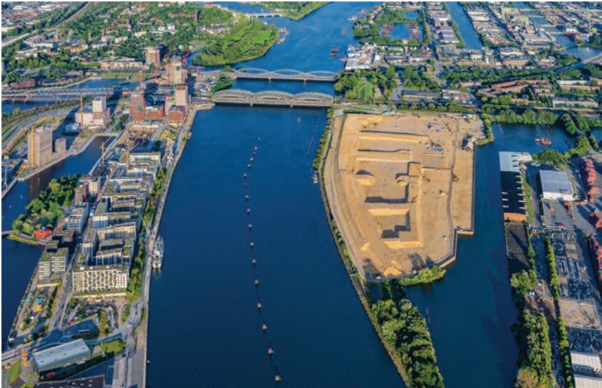
Kleiner Grasbrook (also known as the “Leap across the river” project). Preparation of the site is underway with terps (man-made mounds for flood protection) for buildings and streets. To its left is the final phase of HafenCity development. Image: Martin Elsen, Mediaserver Hamburg
